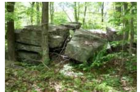
Ortner Drive: Existing stone drainage structures at a section of an abandoned road that bridges an inland wetland and that makes a wonderful trail. (photo: Kristin Elliott Leas)
